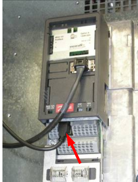
Figure 10. USB cable connected to control card.
