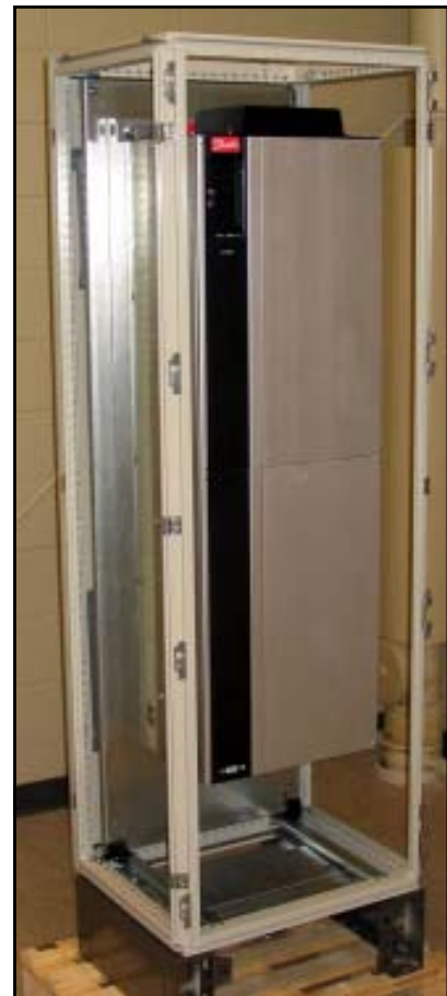
Figure 10. Drive installed in cabinet—D4 Frame
