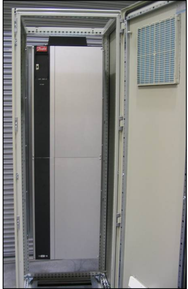
Figure 11. Drive installed on mounting plate
