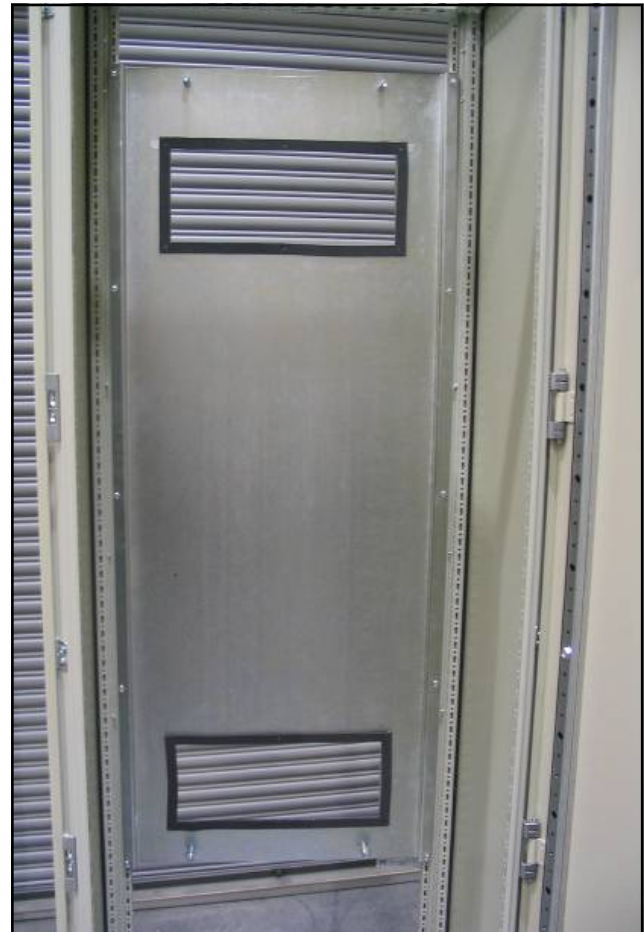
Figure 8. Drive mounting plate installed with rear panel of enclosure removed
