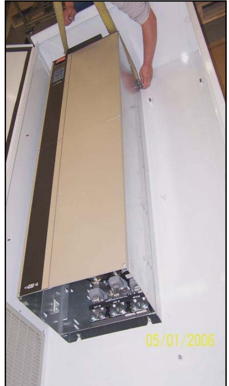
Figure 9. Drive installed in enclosure
